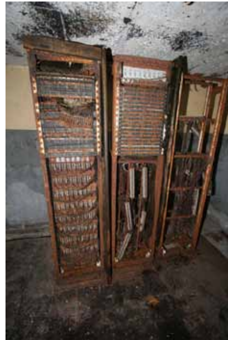
Swichboard in Battery 210 (Chris Zeeman)
