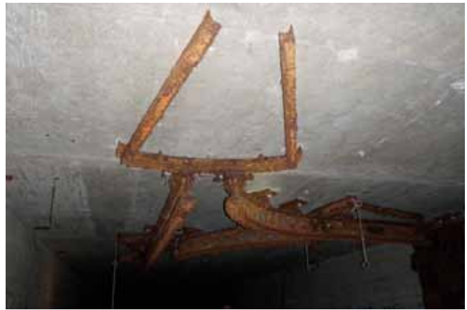
Overhead rails in Battery Gray (Chris Zeeman)
