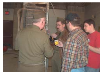
Shawn Welch, Jonathan Prostak, Mike Murray and Stephen Turner working on the BD-74 Fire Control Switchboard.
